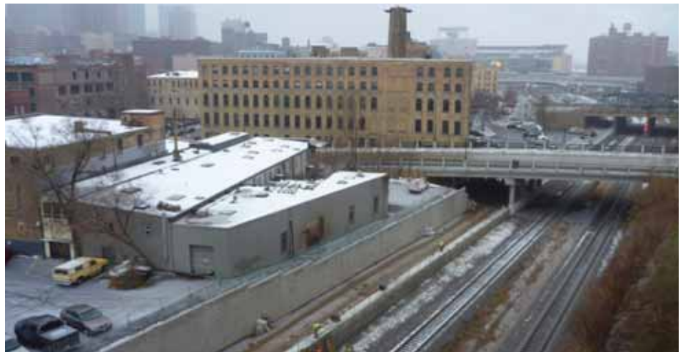
Construction continues even in the snow, with new retaining walls and pavement being installed. Looking west past Washington Avenue and beyond.
